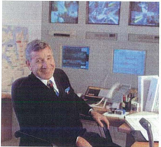
The Metro Light Rail Control room located in Pyrmont.
