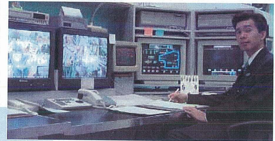
The Monorail central control tower located in Pymont.
