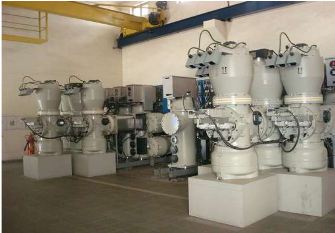
Typical High Voltage Gas Insulated Sub-Station (GIS)
