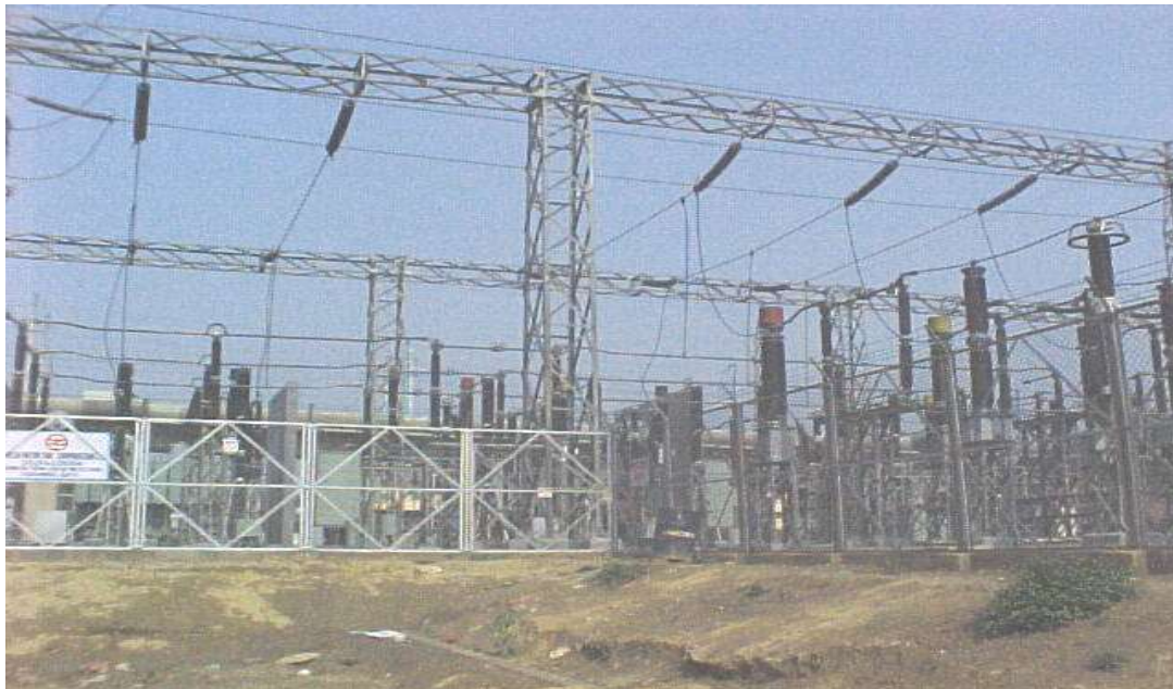
Typical High Voltage Receiving Sub-station
