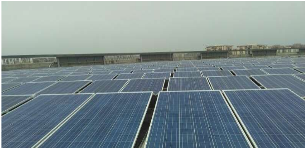
Solar PV Power panel
